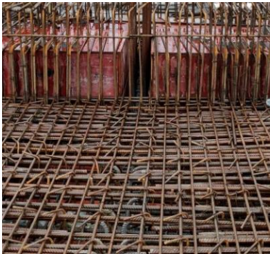
Figure 2. Representative picture of heavy reinforcement taken by the author at a similar construction site.
